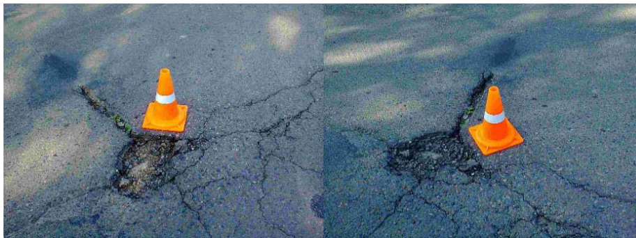
Figure 4. Stereo pair: road cone against the background of damage to the road surface
