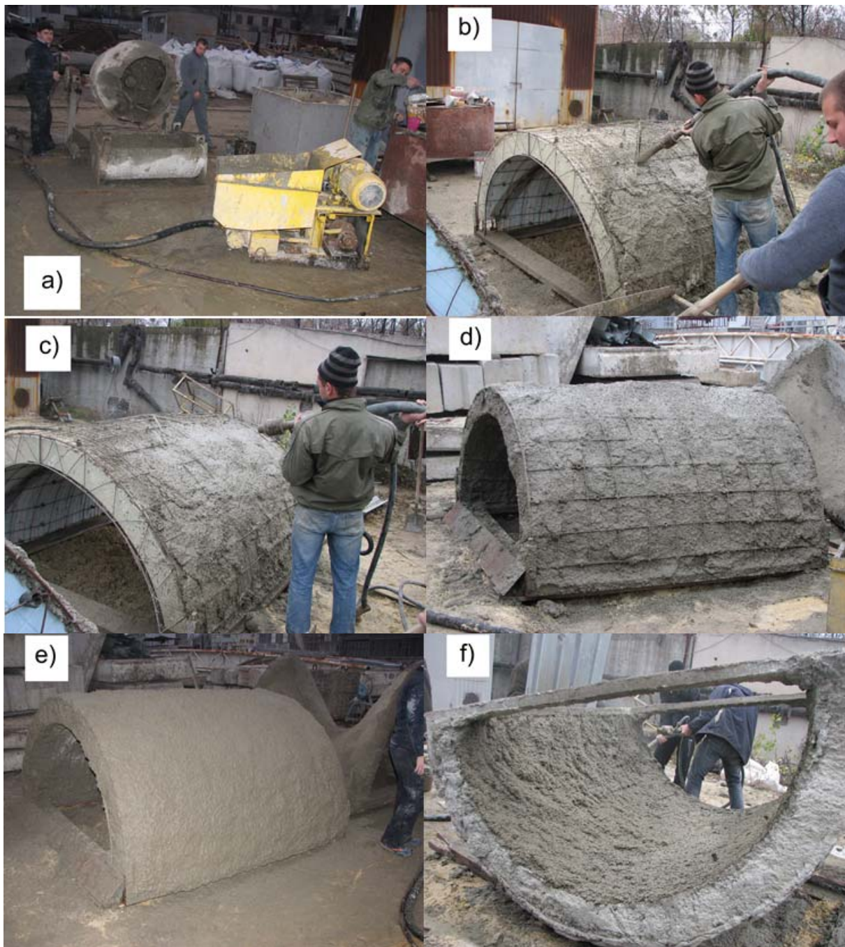
Fig.10 Concreting process of cast reinforced concrete shells: a) spraying plant, b) seams filled; c) external cladding sprayed; d) first concrete layer sprayed on frame from outside; e) appearance of sprayed concrete before deposition of finish layer; f) internal cladding sprayed
