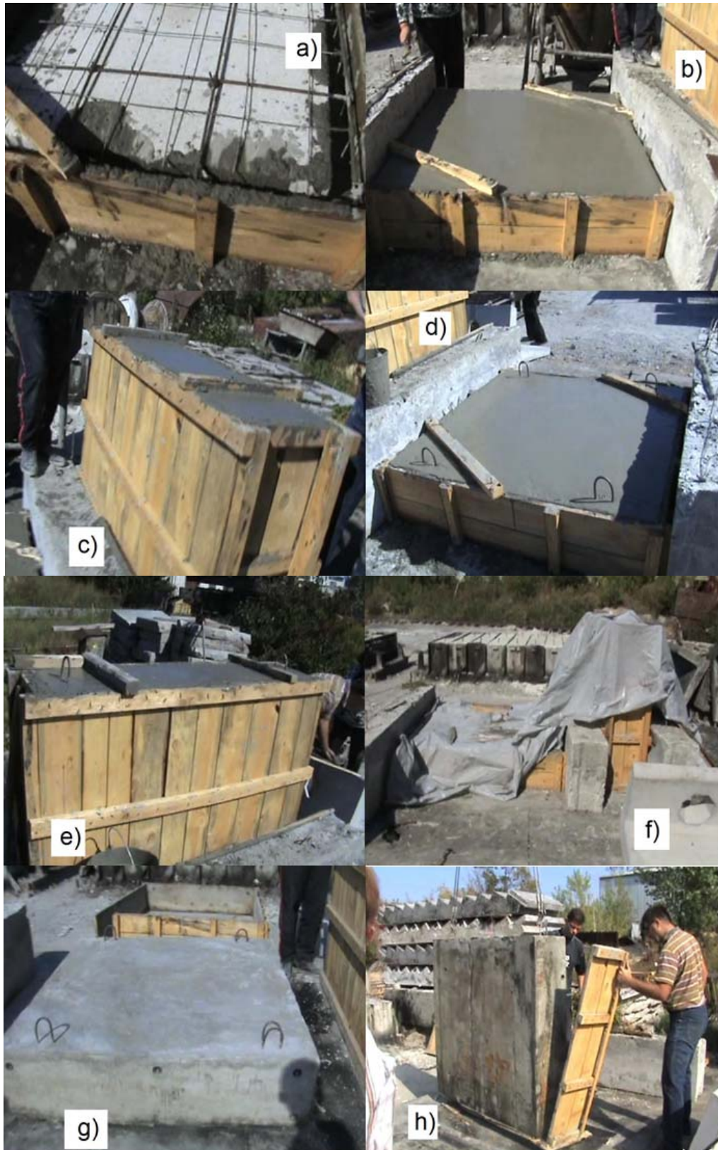
Fig.16 Concreting of lightweight structures using self-compacting concrete in one stage and two layers: a) placing first mortar layer below insert; b) placing second layer for horizontal element; c) placing second layer for vertical element; d) installation of erection loops for horizontal element; e) installation of erection loops for vertical element; f) shrouding of concreted structures with film for concrete to gain strength; g) stripping of formwork from horizontal element; h) stripping of formwork from vertical element
