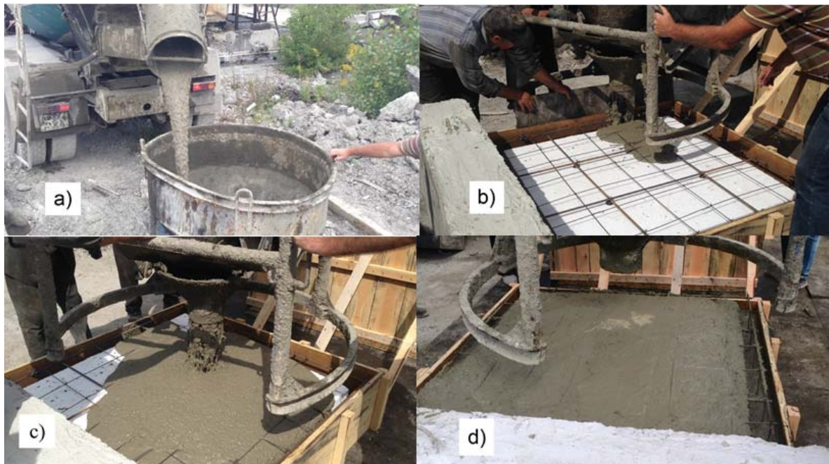
Fig.14 Concreting of lightweight structure horizontal element: a) loading of self-compacting concrete mortar to bucket; b) mortar placing to form slab bottom cladding below insert; c) mortar placing to form ribs and slab top cladding; d) floating-up of concrete fabric together with insert
