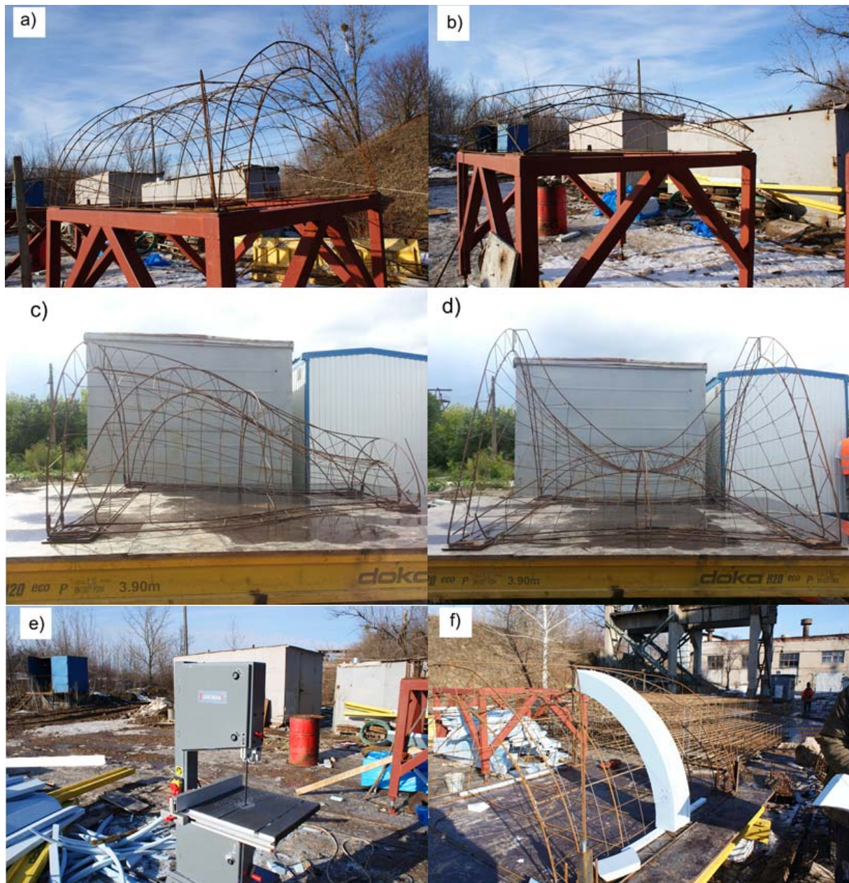
Fig.8 Elements of self-bearing frame for concreting of reinforced concrete shells: a) frame elements for cylinder fragments; b) frame elements for sphere fragments; c) frame elements for nodoid fragments; d) frame elements for hyperbolic paraboloid fragments; e) foam polystyrene sheet cutting machine; f) process of insert installation within frame
