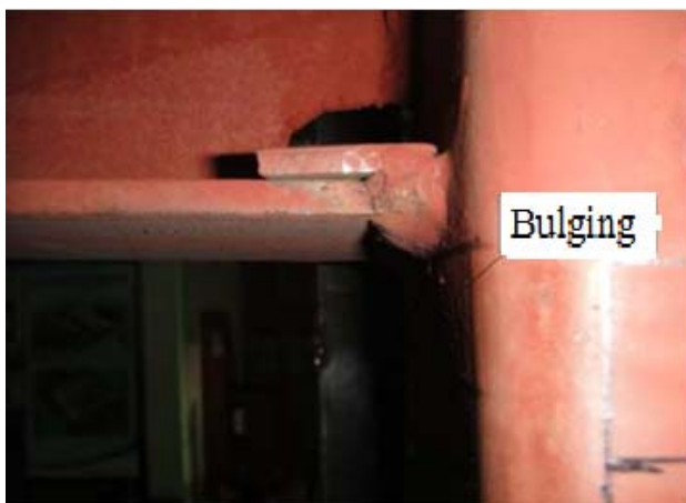
(c) Bulging of the column
