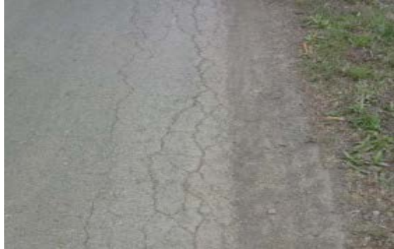
Fig.4 (a) Core sample 2 original pavement
