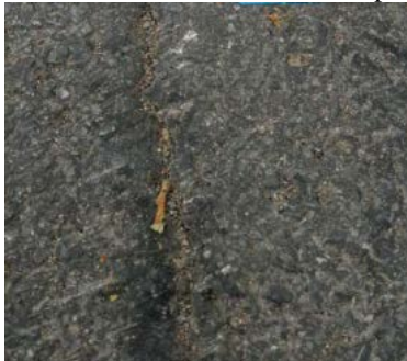
Fig.3 (a) Core sample 1 original pavement
