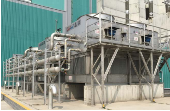
Figure 1. HVDC converter valve substation applied with closed circuit cooling towers
