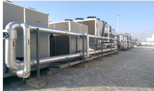
Figure 6. Photo of air cooler series with the air-cooled chiller system
