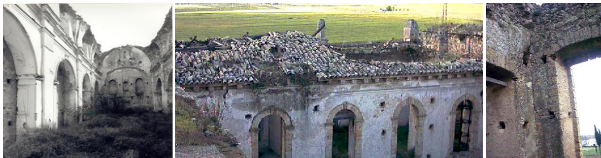
Figure 14: Conservation status of the Church of the Friary: internal view (on the left); ruins of ancient roofing, now collapsed (in the center); detachment of the internal walls from façade walls (on the right)
