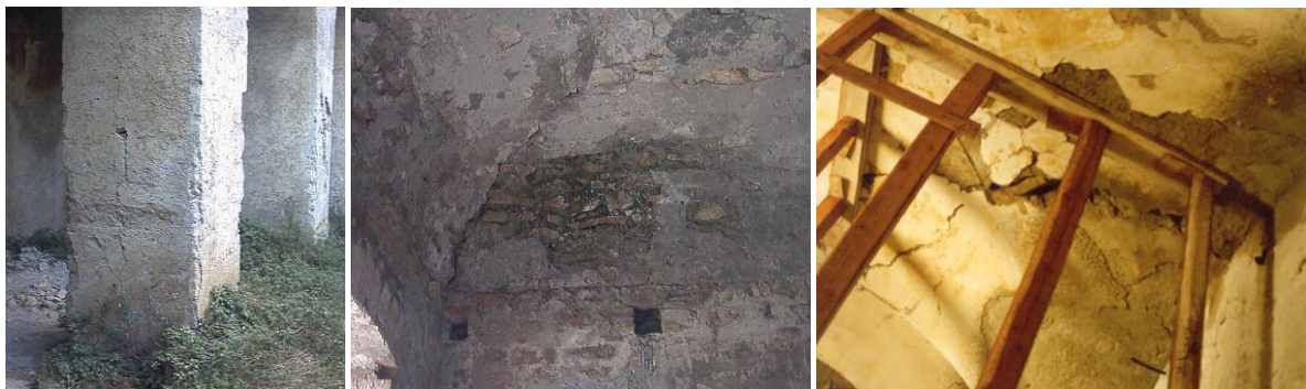
Figure 13: Degradation of the cloister's structures: pillar damaged by crushing (on the left); vaults remaining at the ground floor (in the center); vaults nearly collapsed (on the right)
